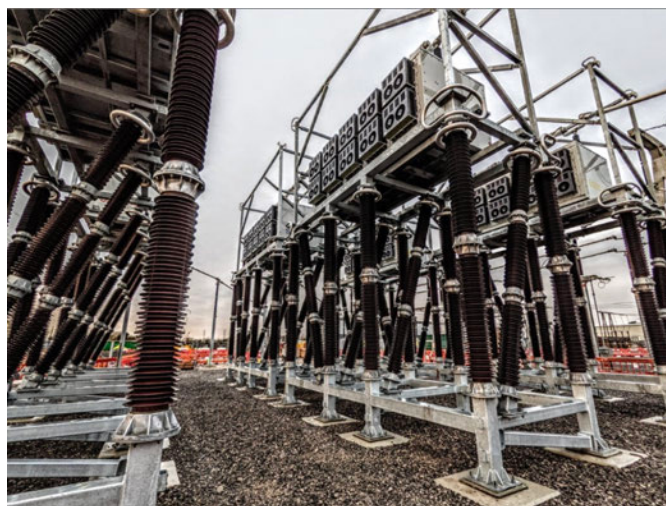
Figure 5: Smartwires deployed at a UK substation
