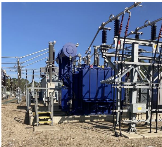
400kV Synthetic Ester Filled Transformers (NIA_NGET0080): Has led to us adopting synthetic ester in large power transformers. These types of transformers (identified by their blue colour) are installed across multiple substations and continue to be used where required. Lifetime savings for installing synthetic ester transformers as opposed to traditional mineral oil transformers are approx. ██████ per transformer. We have 22 synthetic ester transformers either built or in active construction (9 deployed, 13 under construction) which equates to a ██████ cost reduction and therefore consumer benefit. This benefit is in addition to wider benefits from synthetic ester transformers including: environmental benefit vs traditional mineral oil, reduced CO 2 , reduced onsite footprint, predicted longer life for transformer, option to provide community heating from waste heat.
