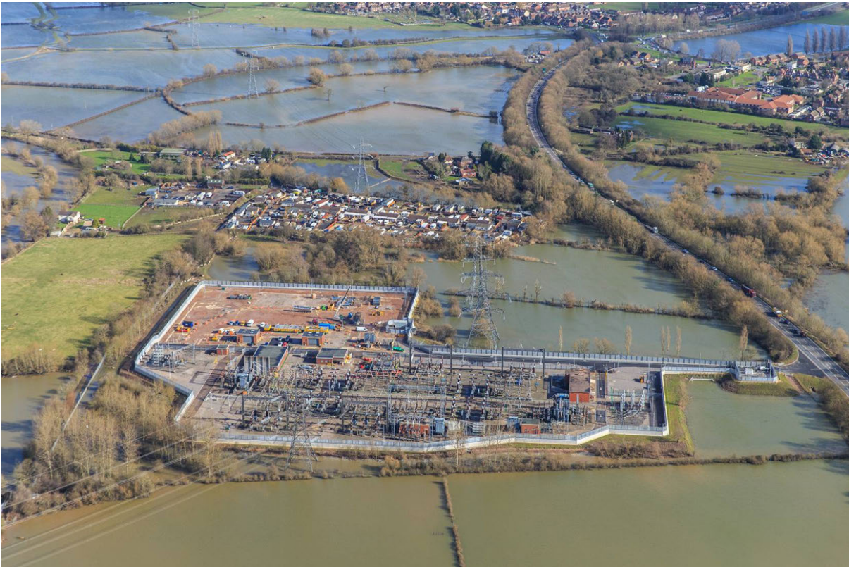
Figure 4: NGET Walham substation protected by flood defences
